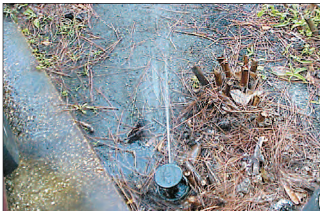
Figure 10. Object is interfering with spray pattern, resulting in poor distribution uniformity
