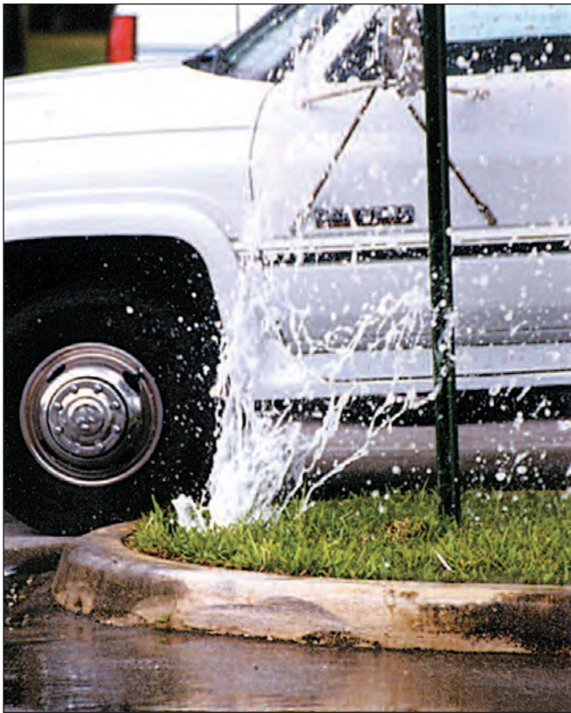
Figure 11. Water gushing from broken head.
