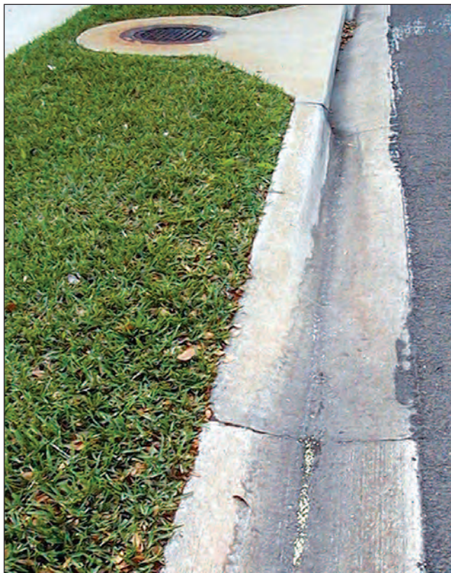
Figure 19. Slow or quick release, this fertilizer is going to a water body. Keep fertilizer away from impervious surfaces and water bodies.
